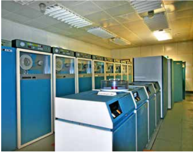
Control room for life support and plant. Photo Tim Wellburn
